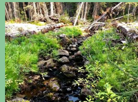
Inspection of a recent bridge deactivation project at the Company's Fort St. James operation found that the operation had done a good job of protecting the stream channel during the deactivation of the crossing.
