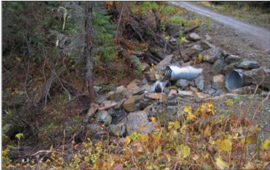
Photo depicting armouring of culvert discharge area and diversion of runoff into vegetated area where it can be filtered.
