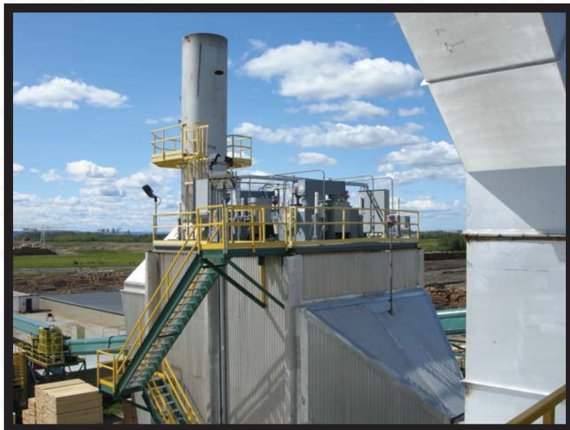
Fort St. John Energy System - Fort St. John, B.C.
