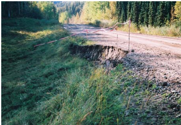
Figure 11. Slump on Waskahigan Mainline
