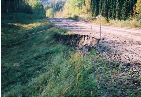
Figure 10. Slump on Waskahigan Mainline
