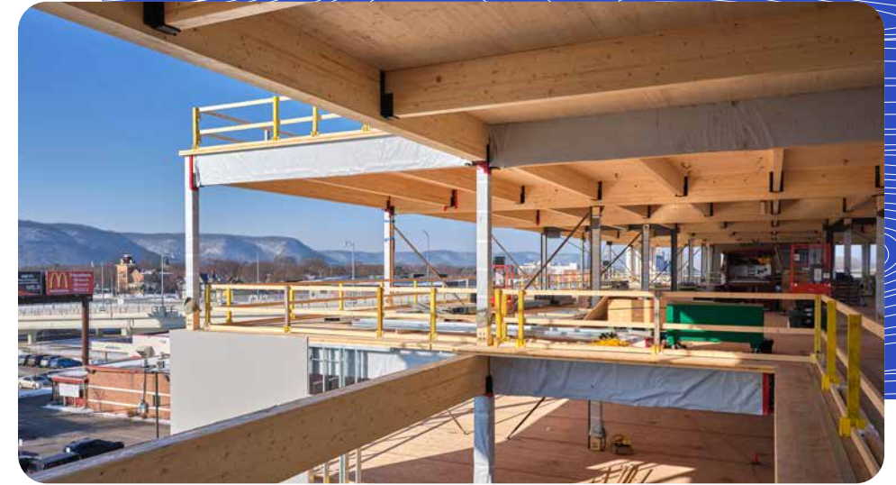
Mass timber building construction including Canfor lamstock. Photo credit: ©The Kubala Washatko Architects. Photo courtesy of Western Archrib.
