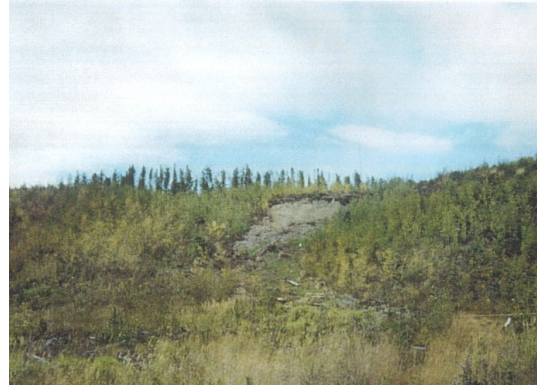
Figure 9. Minor Slump in Block W73067
