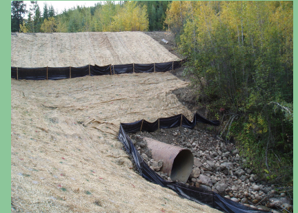
Sediment control measures were found to be effectively implemented to protect water and fisheries resources.
