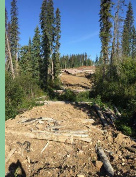
This photo shows a temporary winter road where it crossed a watercourse. The bridge has been removed, and visible at the centre of the frame is the intact riparian vegetation. The road surface has been decompacted and will be grass seeded and planted. The log pieces on the former road surface visible in the foreground have been placed to interrupt sediment movement.
