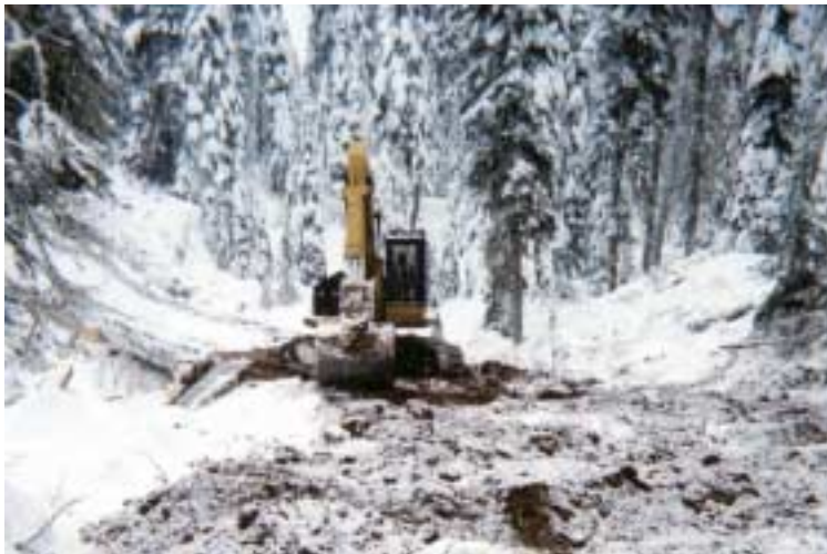
Equipment operators and foreman continue to show a high level of awareness of environmental and site-specific issues during road and bridge construction on TFL 30.
